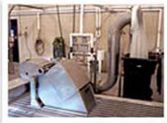
Fine Step Screen, Wash Press, & Hygienic Bagger (Assumption WWTP, QC)
