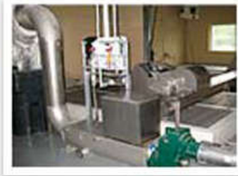
Wash Press Screw Compactor (Assomption WWTP, QC)
