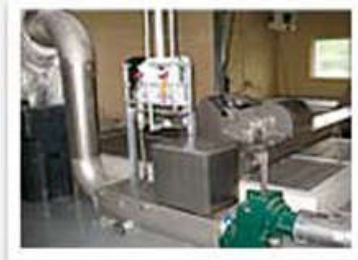
Wash Press Screw Compactor (Assumption WWTP, QC)
