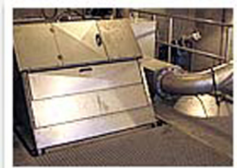
Fine Step Screen and Wash Press (Repentigny WWTP, QC)
