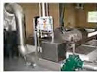
Wash Press Screw Compactor (Assumption WWTP, QC)
