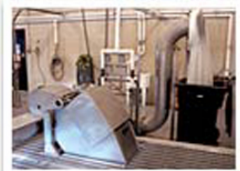
Fine Step Screen, Wash Press, & Hygienic Bagger (Assomption WWTP, QC)
