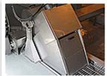
Fine Step Screen and Shaftless Screenings Transfer Conveyor
