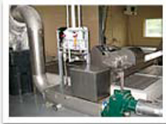
Wash Press Screw Compactor (Assomption WWTP, QC)
