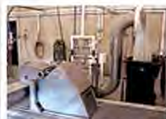
Fine Step Screen, Wash Press, & Hygienic Bagger (Assumption WWTP, QC)
