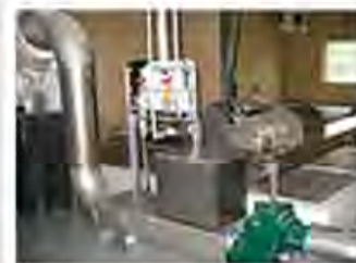
Wash Press Screw Compactor (Assomption WWTP, QC)
