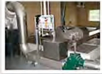
Wash Press Screw Compactor (Assumption WWTP, QC)
