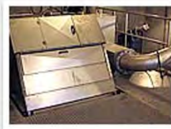
Fine Step Screen and Wash Press (Repentigny WWTP, QC)
