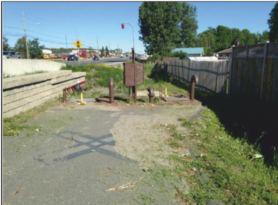
Photo 10: Kingsway Lift Station Wet well / vents and electrical / instrumentation structure contains visually similar paint to sample 1955Ki-Ex-P-03 – Entrance Door (Brown) - Result - <98 µg/g (<0.0098%) above
