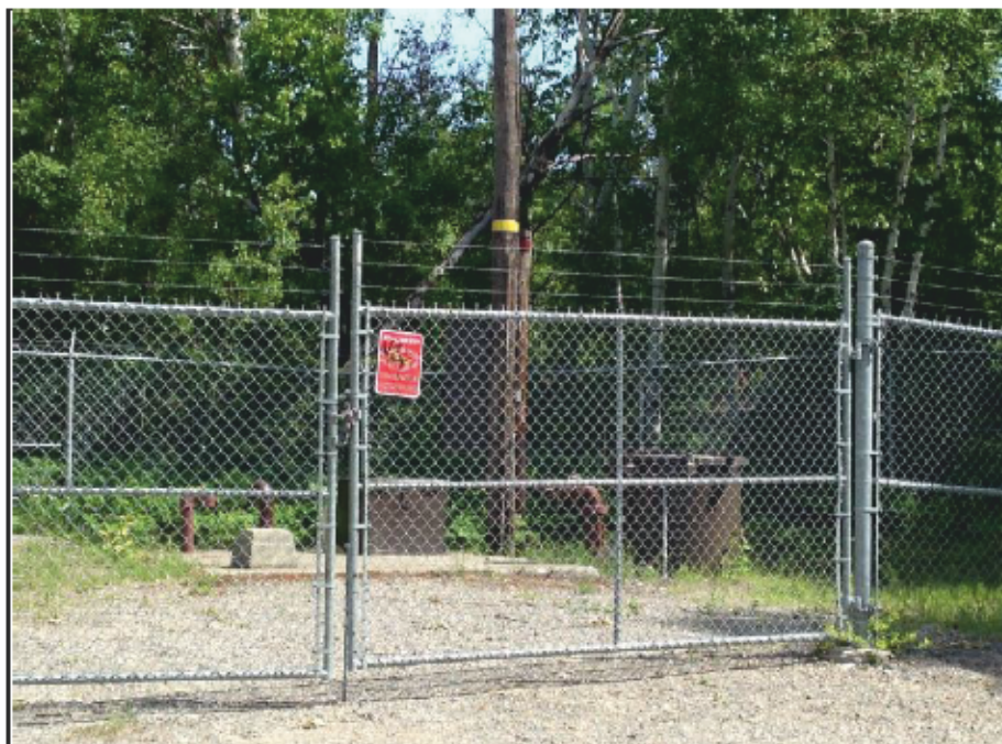
Photo 12: Hudson Rd. Lift Station – Exterior brown paint on associated wet well / vents and electrical / instrumentation structure contains visually similar paint to sample 1955Ki-Ex-P-03 – Entrance Door (Brown) - Result - <98 µg/g (<0.0098%)
