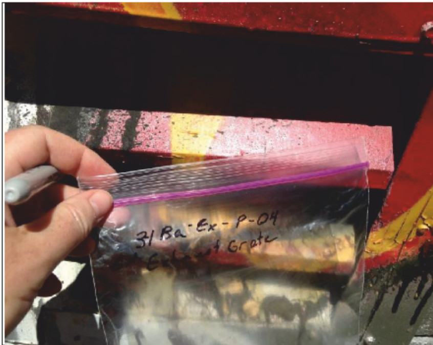
Photo 4: Bancroft Drive Lift Station Sample # 2811Ba-Ex-P- 04 – Vent (graffiti mix) - <math>120 \mu\text{g/g}</math> (0.012%) lead by dry weight – Condition – Very Poor
