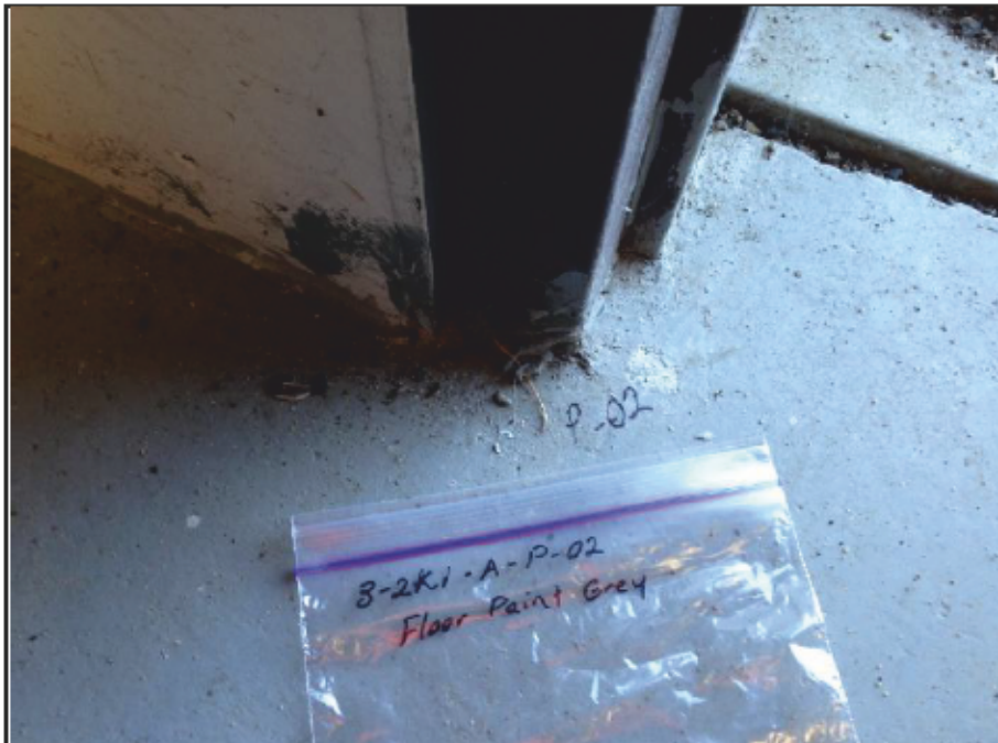
Photo 8: Kingsway Lift Station Sample # 1955Ki-A-P-02 - Floor (grey) - Result - <91 µg/g (<0.0091%) lead by dry weight - Condition - Fair
