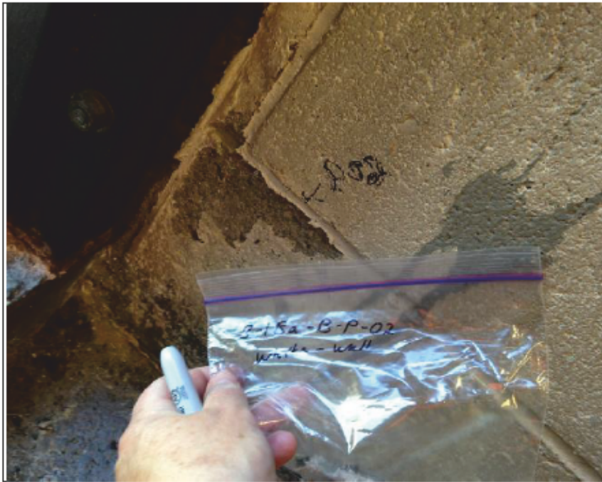
Photo 3: Bancroft Drive Lift Station Sample # 2811Ba-B-P-02 – Walls and ceiling (white) - <math>68 \mu\text{g/g}</math> (0.0068%) lead by dry weight – Condition – Poor
