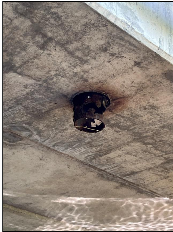
Photo 15 – Severe corrosion with perforations and section loss typical in deck drains.
