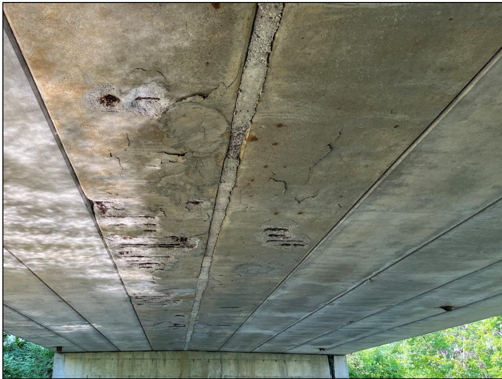
Photo 13 – Severe spalls with exposed corroded reinforcement and delaminated areas along entire length of two girders at centerline of structure.
