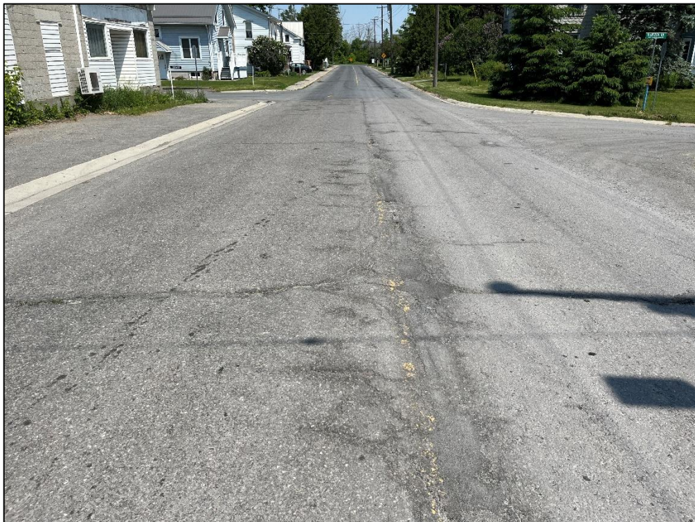
Photo 4 – Severe alligator cracking and loss of patching material in approach wearing surface resulting in severe potholes.
