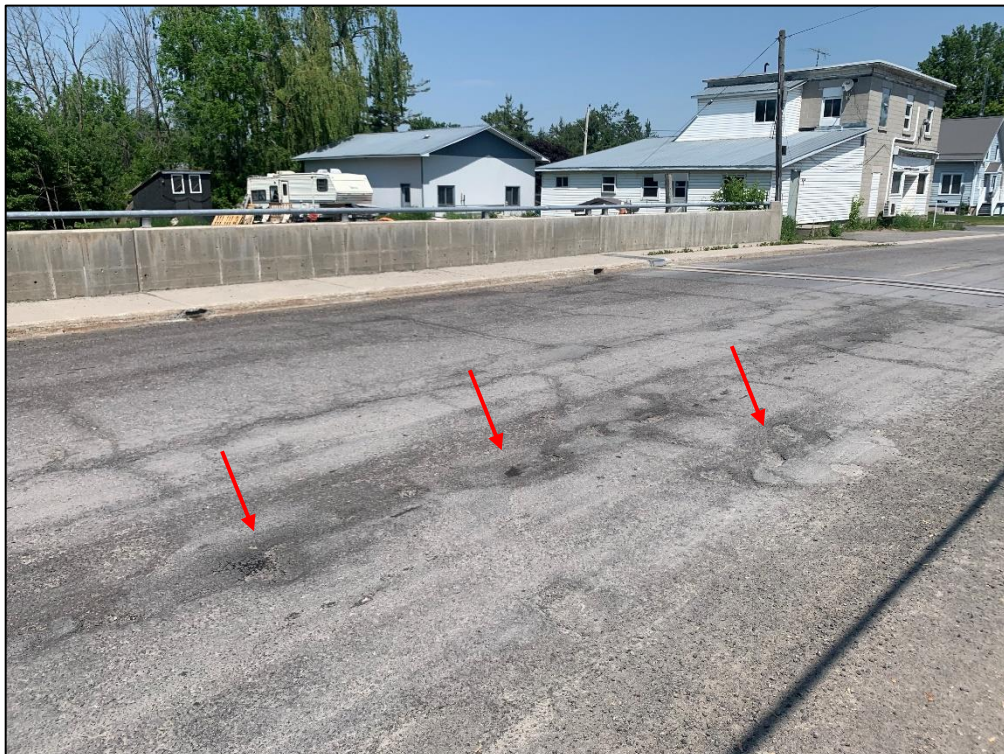
Photo 6 – Severe map cracking throughout deck wearing surface. Severe potholes in northbound lane.
