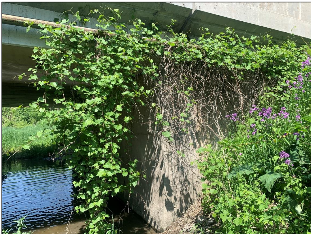
Photo 16 – Excess vegetation encroaching on wingwall and conduit at northeast quadrant.
