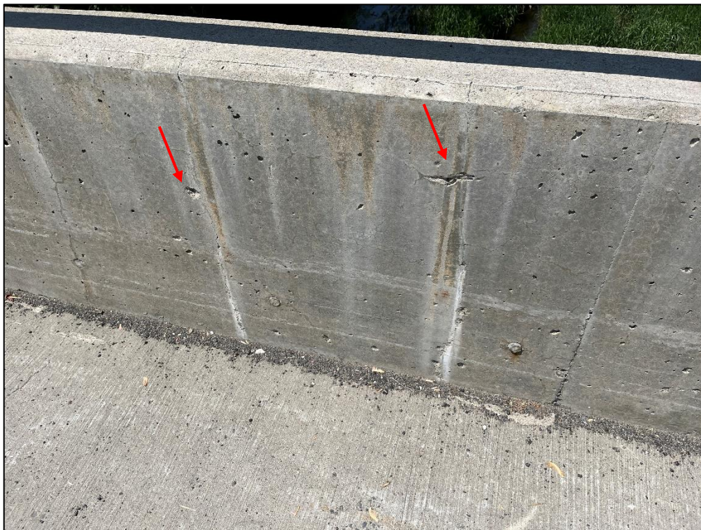
Photo 8 – Small localized spalls typical along east and west parapet wall interior.
