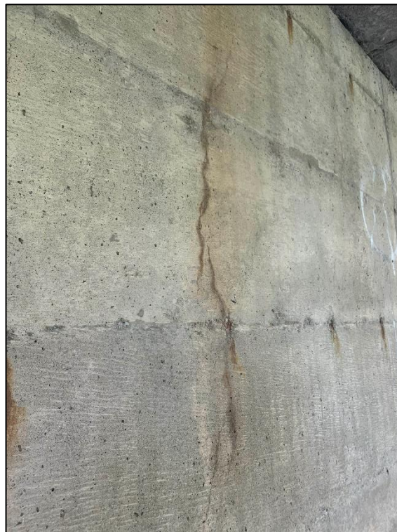
Photo 14 – Hairline to narrow vertical cracks with wet staining on south abutment wall.
