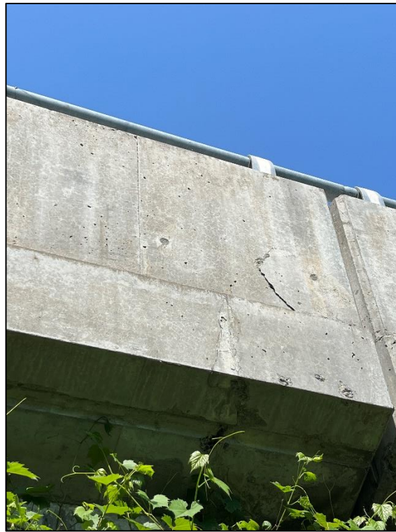
Photo 9 – Severe delamination along east parapet wall exterior.
