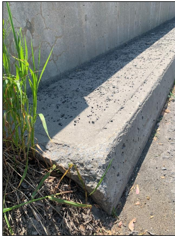
Photo 11 – Spall at north end of east curb.
