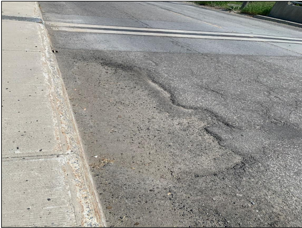
Photo 7 – Very severe raveling and loss of asphalt in northwest corner of deck wearing surface.
