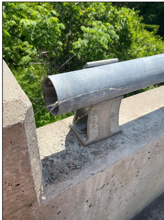
Photo 10 – Missing end cap at northeast end of hand railing.
